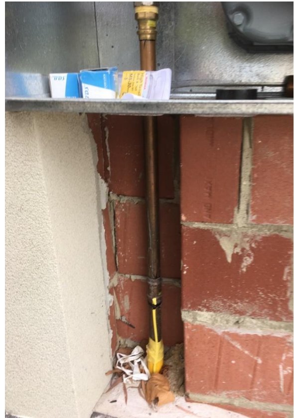
Non-conforming Installation (Surface is not finished, not sealed, and cracks in the brickwork, which provide a leak path to the cavity)
