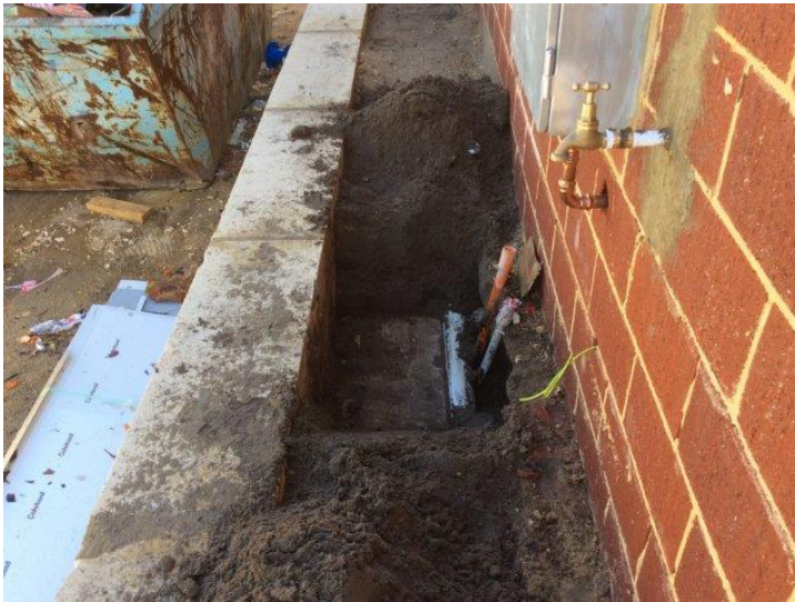
Figure 14: Non-compliant Service Separation (Less than 150 mm between Utilities)
