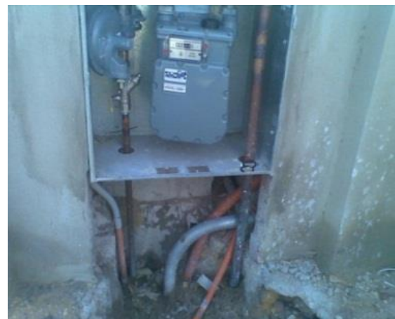
Non-conforming Installation (Other Services Installed)
